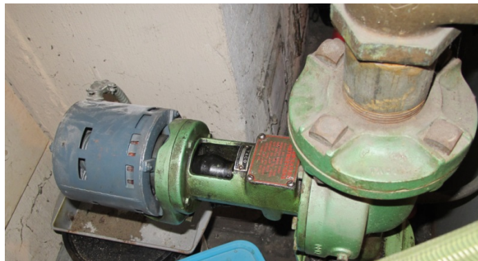
Figure 16. Primary circulator at Building B
