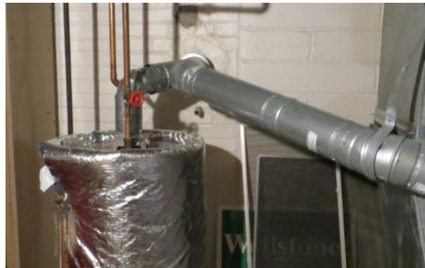
Figure 9. Common vented water heater
