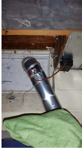
Figure 7. Custom wireless sensor module (black box) with pressure sensing tube placed in dryer exhaust duct
