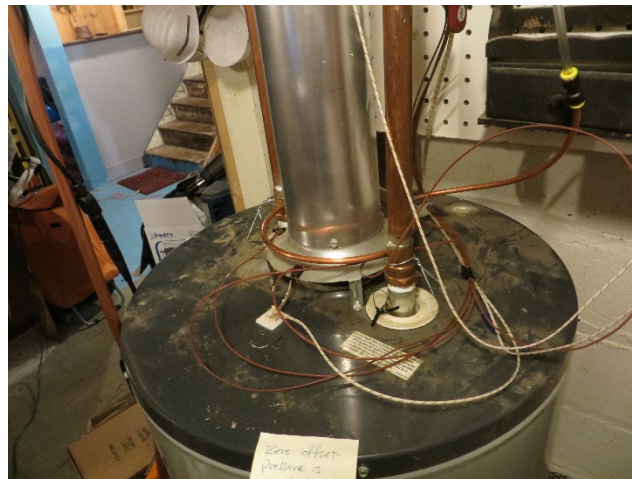
Figure 6. Water heater draft hood with copper tube for CO 2 sampling and thermocouple temperature wire showing
