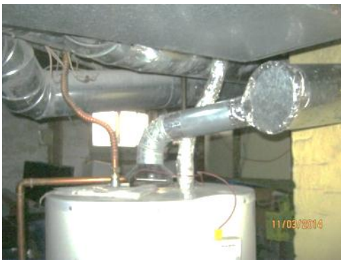
Figure 8. Orphaned water heater
