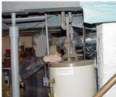
Figure 1. Checking spillage on a water heater
