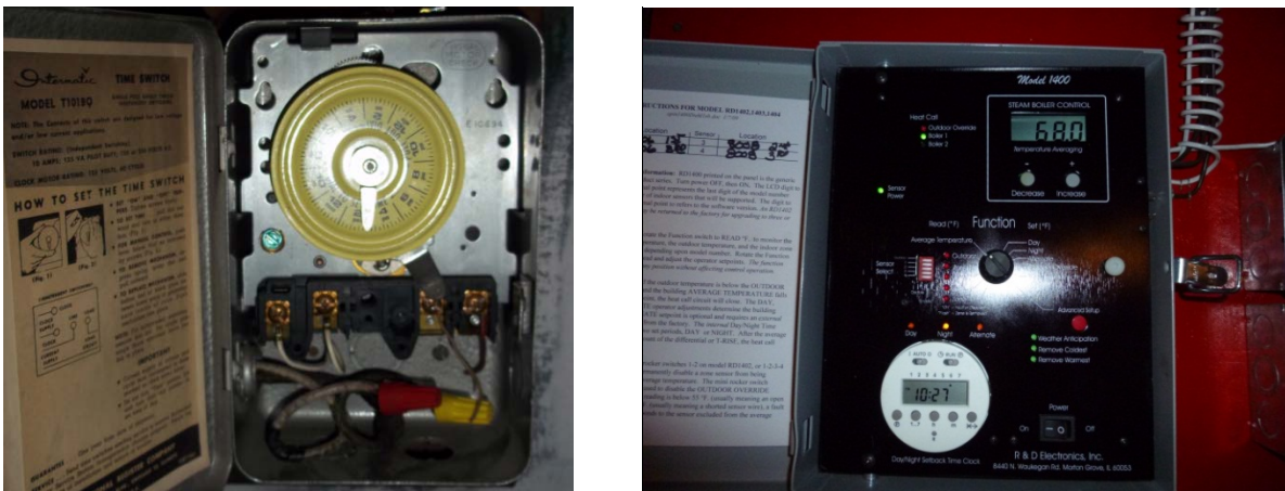
Figure 5. Left: Previous timer control, which operated boiler by signaling it to fire during certain times of the day. Right: New boiler reset control with four remote indoor temperature sensors and one remote outdoor temperature sensor.
