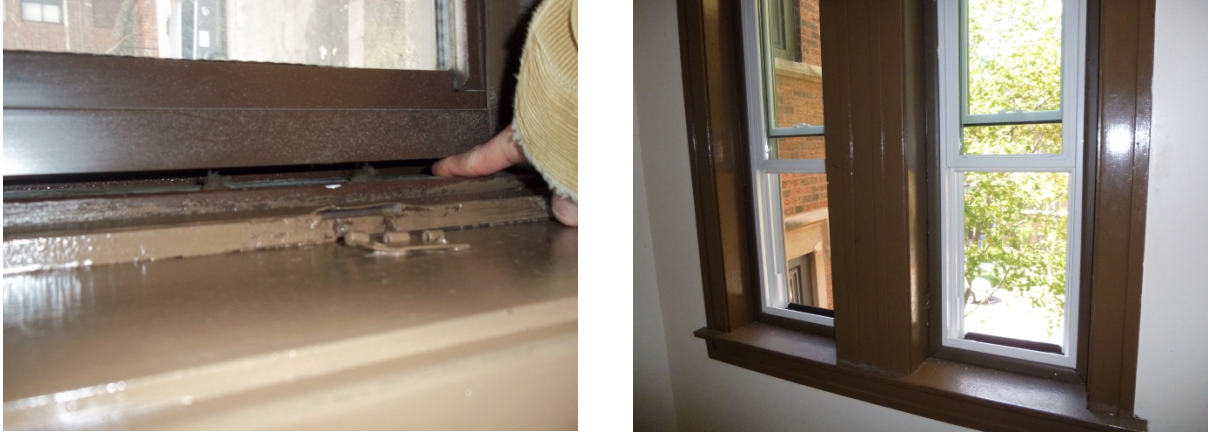
Figure 14. Left: Air gap between window frame and wall. Right: Newly installed windows.
