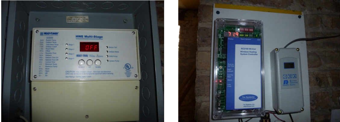
Figure 11. Left: Existing outdoor reset controller. Right: New room temperature averaging control.
