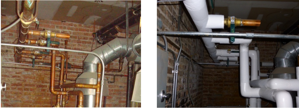
Figure 9. Left: Bare hot water pipes. Right: Pipes insulated with 1 in. jacketed fiberglass.
