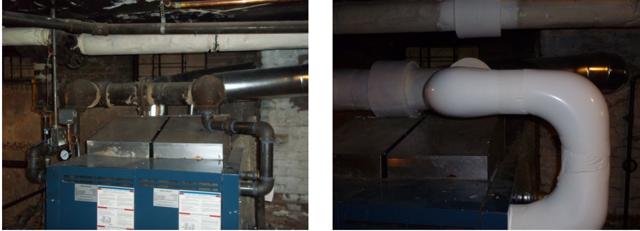
Figure 4. Left: Uninsulated steam piping. Right: Steam pipes insulated with jacketed fiberglass.
