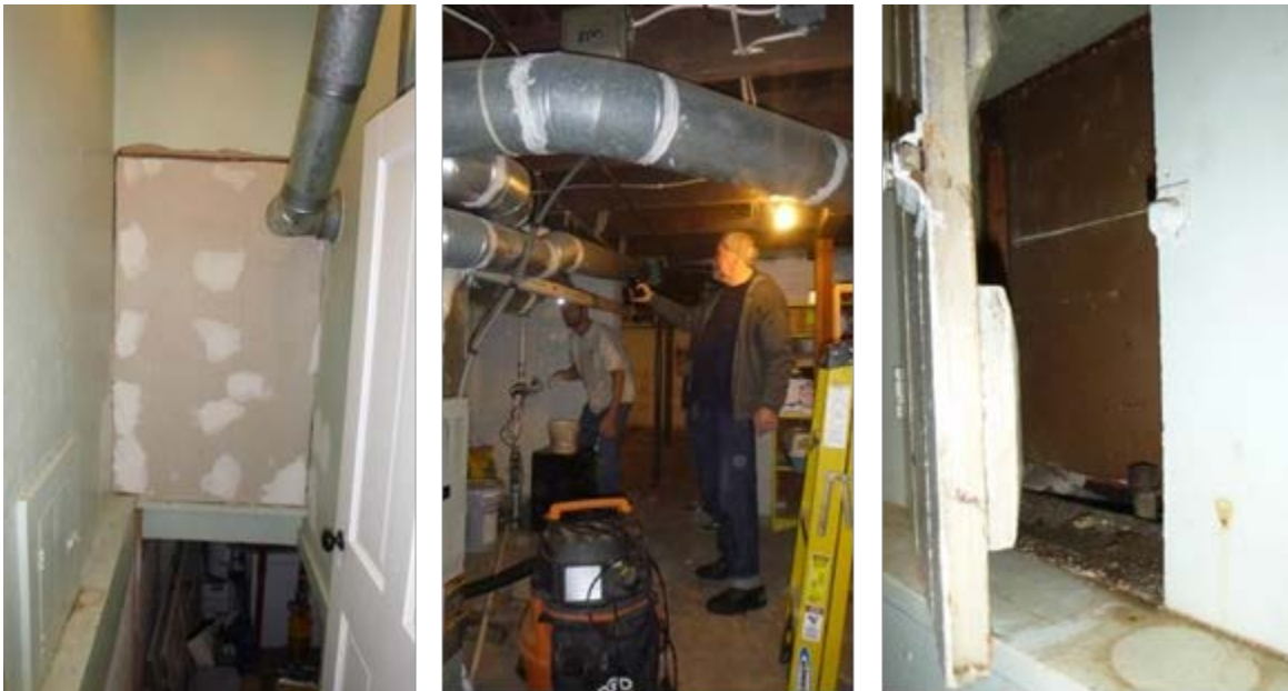
Figure 3. Large bypasses at the basement entry (left); ductwork sealing (center); sealing at an abandoned laundry chute (right)
