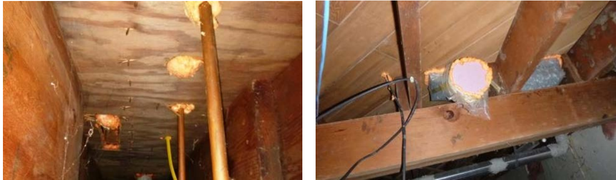
Figure 2. Foam sealing at plumbing penetrations and at supply boot (left); air sealing at ductwork joints (right)
