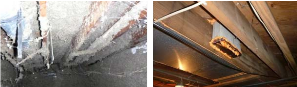
Figure 5. House 5, showing blown cellulose floor system in a crawl space area (left) and ductwork showing a panned return and abandoned riser (right)
