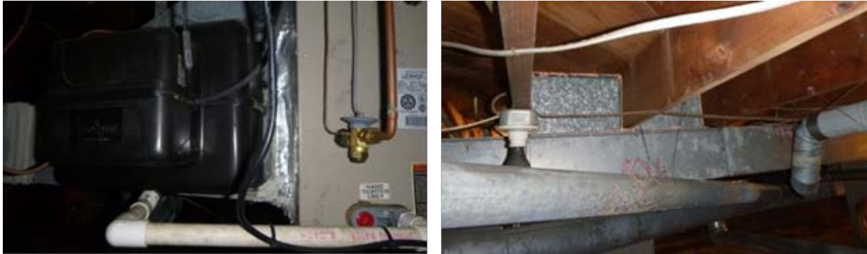
Figure 4. Sealing leakage at the furnace (located in the crawl space) associated with the humidifier (left) and panned return (right)
