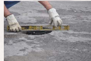
Level Valve Box
