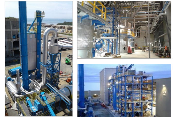
Cote Nord, Quebec, 10M gpy commissioned 2018
