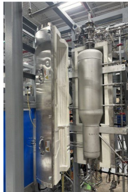
Primary RCFP Reactor
