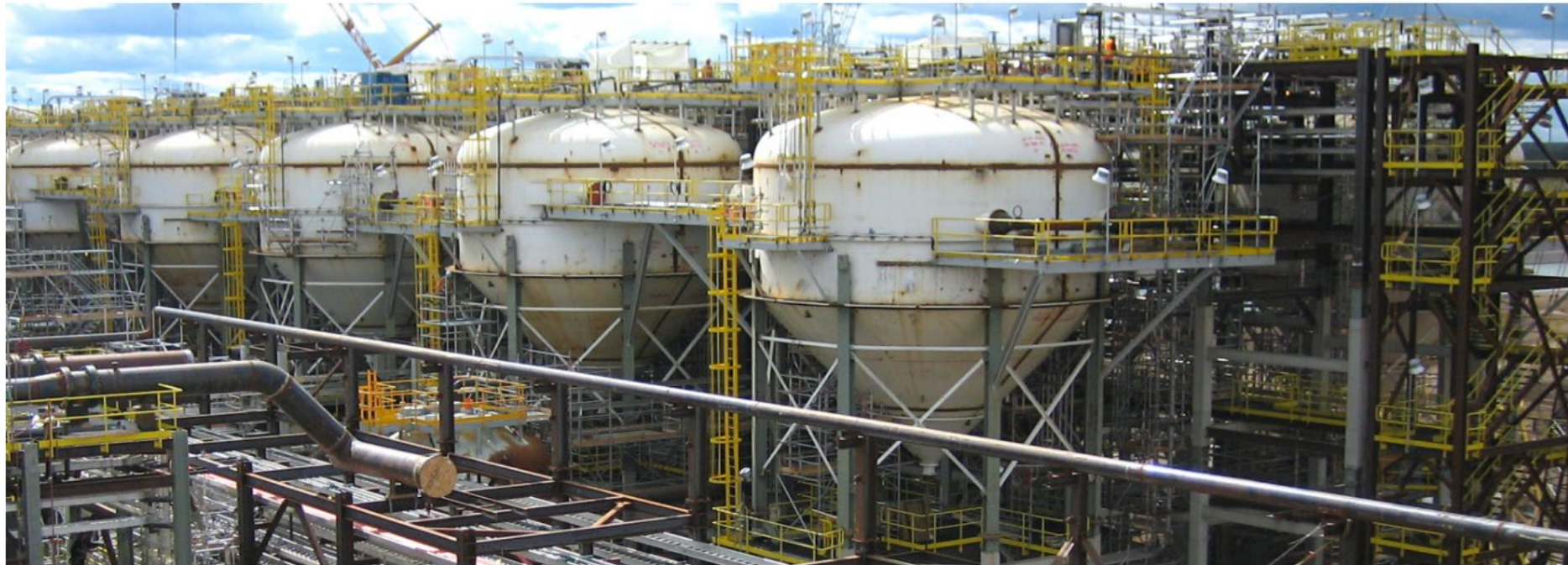
INCLINED PLATE SEPARATORS UNDER CONSTRUCTION AT THE HORIZON FROTH TREATMENT FACILITY (PHOTO COURTESY CANADIAN NATURAL RESOURCES)
