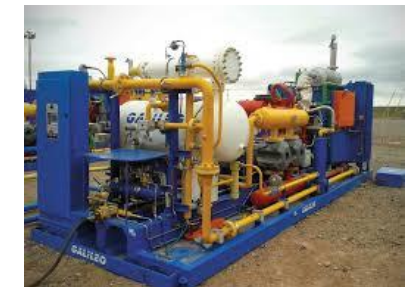
Natural Gas Compressor
